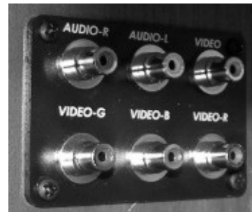
Interior Connection for Satellite Dishes (Located in cabinet near TV)
