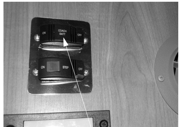
House/Coach Battery Disconnect Switch (Located near entrance door or end of galley, depending on model) -Typical View
