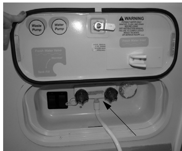
Exterior Shower/Wash Station -Typical View
