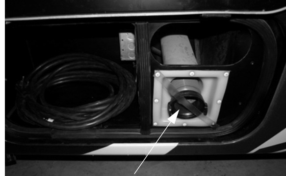
Sewage Drain Hose (Located in utility compartment)
