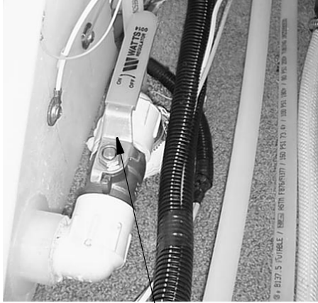
Water Tank Drain Valve (Typical)
