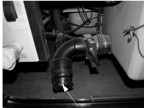
Sewage Drain Outlet/Dust Cap (Located ahead of rear driver side wheel) -Typical View
