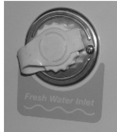
Fresh (City) Water Connection (located inside the exterior wash station)
