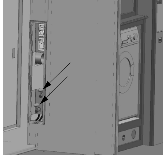
Water Supply Faucets (Located along left-hand side of Stackable Washer/Dryer cabinet - remove panel to access)
