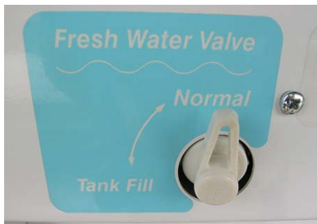
Fresh Water Valve in Normal use position (Located in water service center)
