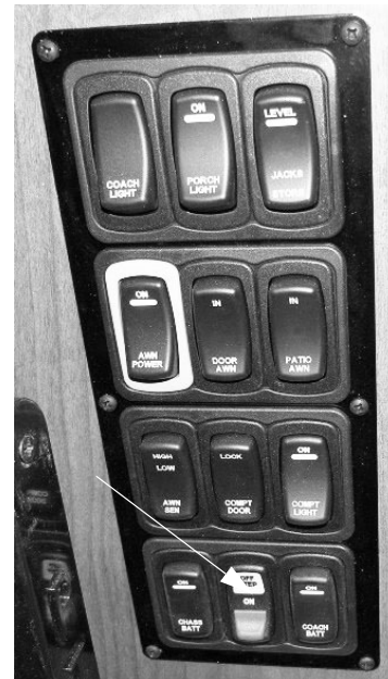
Entry Step Switch (Located near entrance door) -Typical View
