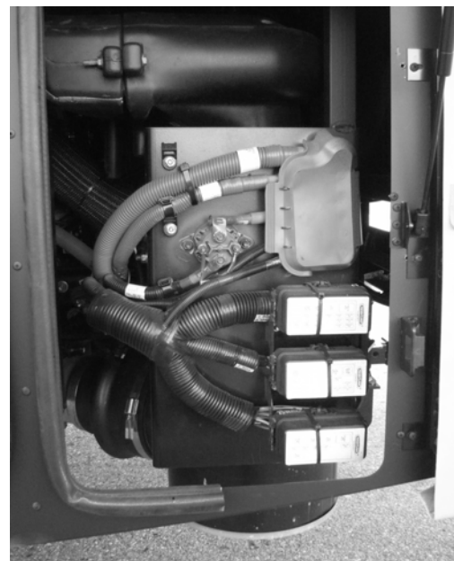
Towing Package Fuses (Located in driver side rear compartment) -Typical View
