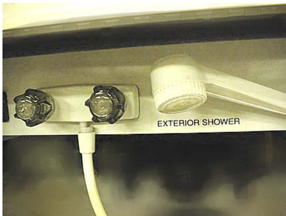
Exterior Shower/Wash Station -Typical View
