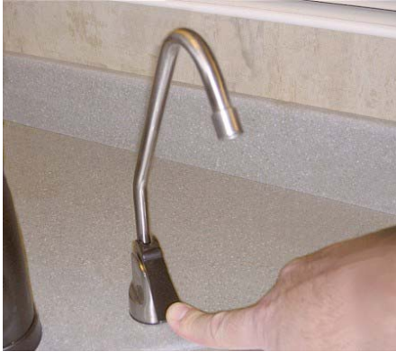
Filtered Water Faucet -Typical View
