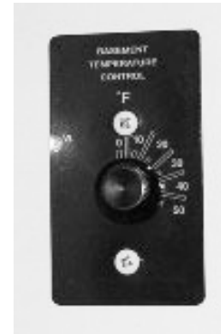
Basement Temperature Control
