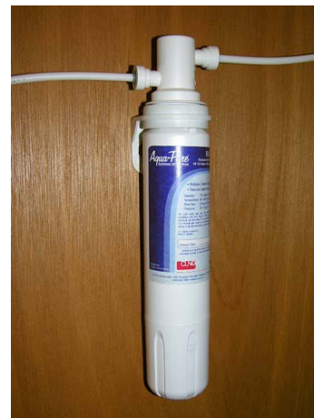
Filtered Water Faucet/Ice Maker Filter Assembly (Located below galley sink)
