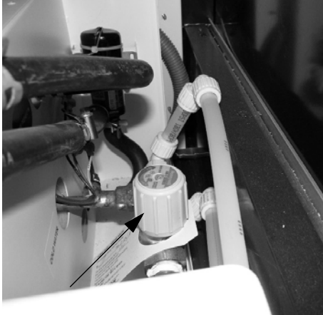
Hydronic Heating System Tempering Valve (Located on back side of the Aqua-Hot unit)
