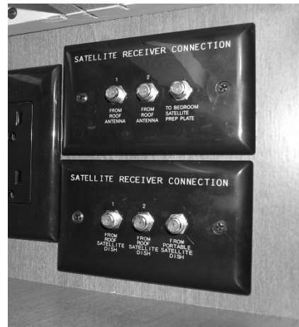
Interior Connection for Satellite Dish (Located near entertainment center cabinet) -Typical View
