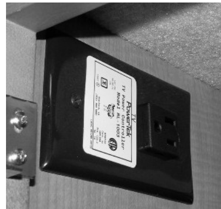
Front TV Ignition Switch Interlock -Typical View
