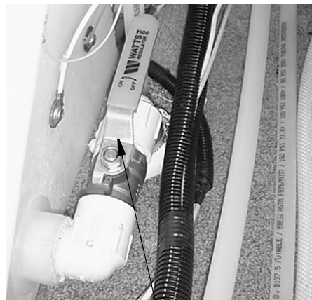
Water Tank Drain Valve (Typical)
