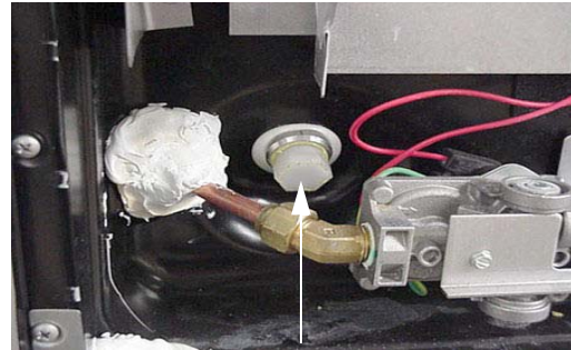
Water Heater Drain Plug (Remove with socket)
