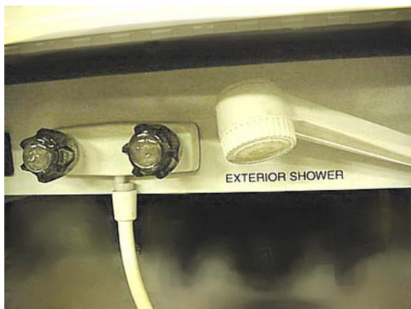
Exterior Shower/Wash Station -Typical View
