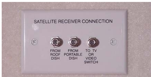
Interior Connection for Satellite Dish (Located in cabinet near TV) -Typical View
