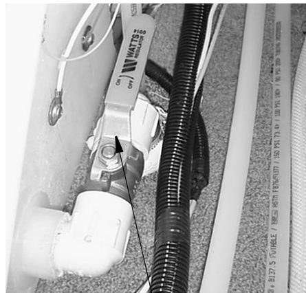
Water Tank Drain Valve (Typical)
