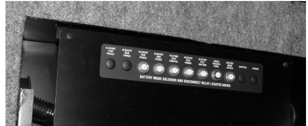
Chassis and House 12V Breakers (Located in passenger side compartment) -Typical View * Shown with cover removed
