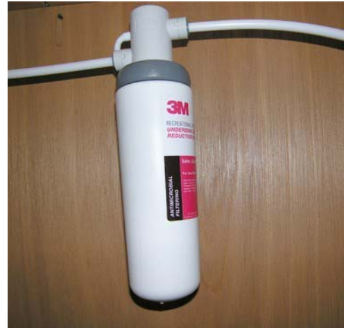
Cold Water Filter Assembly (Located below galley sink)
