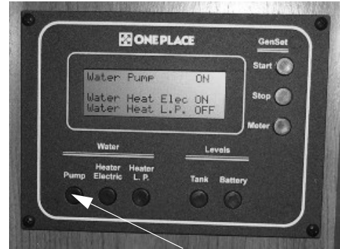
Water Pump Switch
