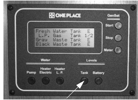
Tank Levels Switch
