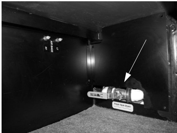
Water Tank Drain Valve (Located in rear driver side compartment)
