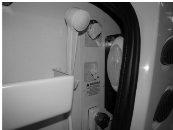
Exterior Shower/Wash Station (Located in backwall exterior service center) -Typical View
