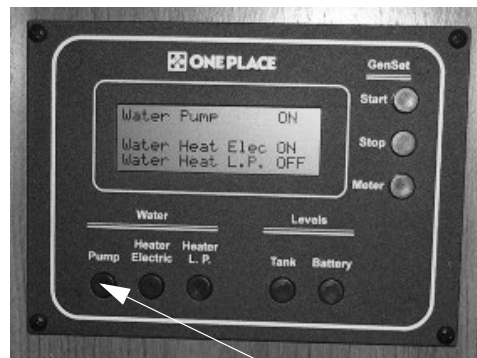
Water Pump Switch
