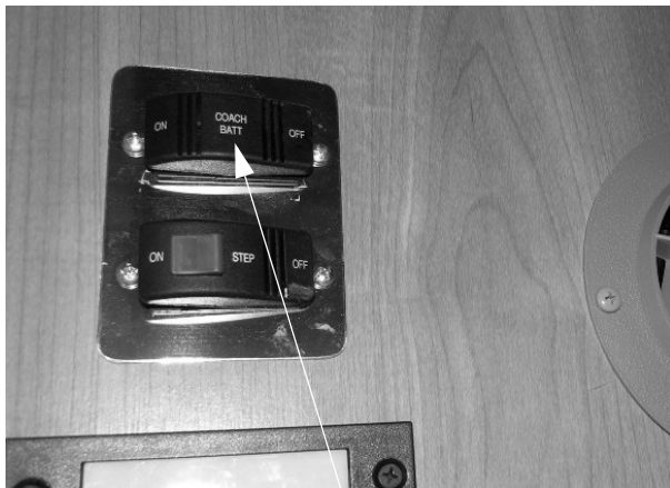
House/Coach Battery Disconnect Switch (Located near entrance door or end of galley, depending on model) -Typical View
