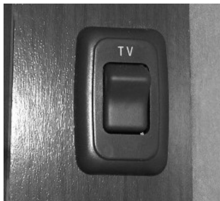
12V TV Master Power Switch (Located on cabinet or wall near TV) -Typical installation shown
