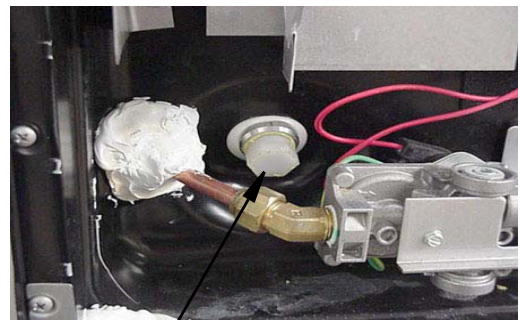
Water Heater Drain Plug (Remove with socket)
