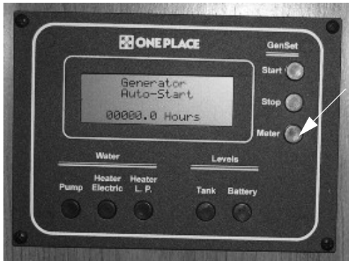
Generator Hourmeter Button -Typical View
