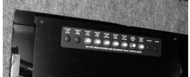
Chassis and House 12V Breakers (Located in passenger side compartment)
