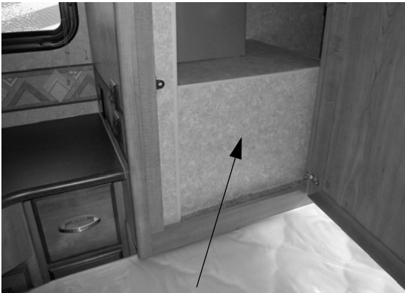
Water Heater Bypass Valve Access (Located within wardrobe - remove front panel to access)
