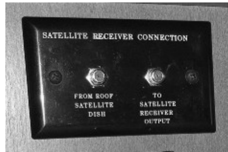
Interior Connection for Satellite Dish (Located near entertainment center cabinet)
