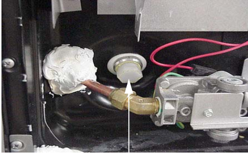
Water Heater Drain Plug (Remove with socket)
