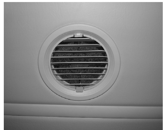
Return Air Vent (Shown with filter installed)
