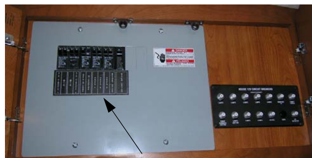
House 120-Volt AC Circuit Breaker Panel
