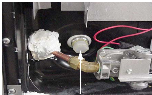
Water Heater Drain Plug (Remove with socket)
