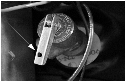
Pressure Temperature Relief Valve (Lift handle only when water heater is cold)
