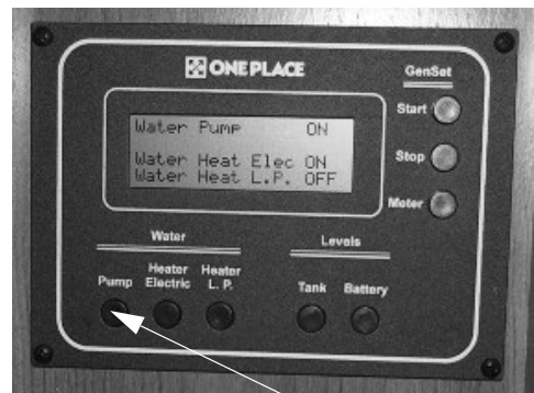
Water Pump Switch
