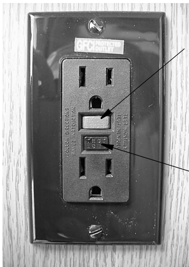
GFCI Outlet (Ground Fault Protector)
