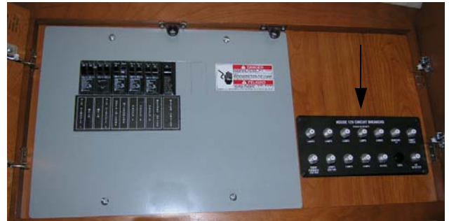
House 12-Volt Circuit Breaker Panel -Typical View
