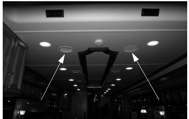
Supply/Return Air Vents (Located throughout the ceiling of the coach) * View looking to rear of coach
