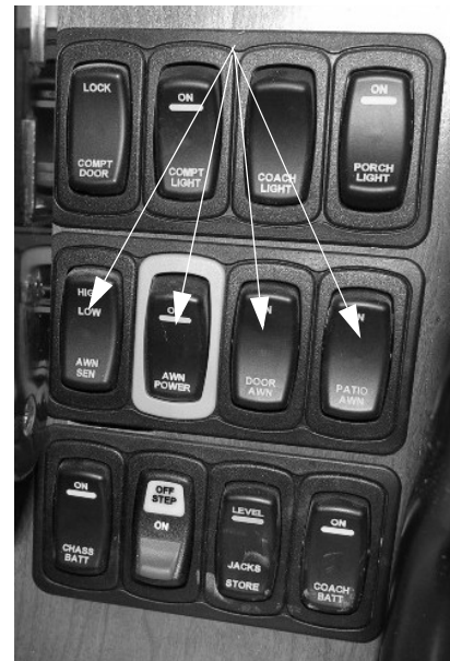
Awning Control Switches (Located near entrance door) -Typical View
