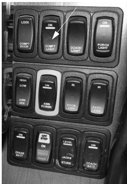
Compartment Lights Switch (Located near entrance door) -Typical View
