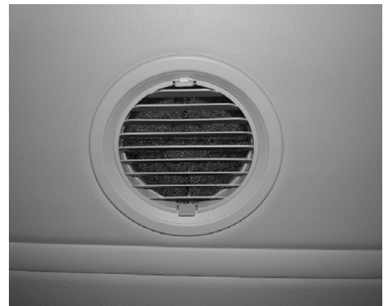
Return Air Vent (Shown with filter installed)
