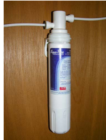
Water Filter Assembly (Located below galley sink)
