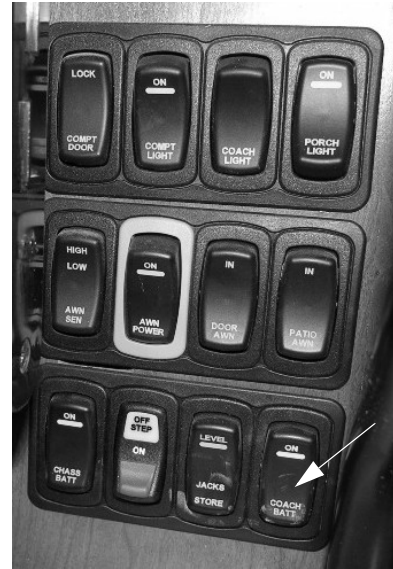
House/Coach Battery Disconnect Switch (Located near entrance door) -Typical View
