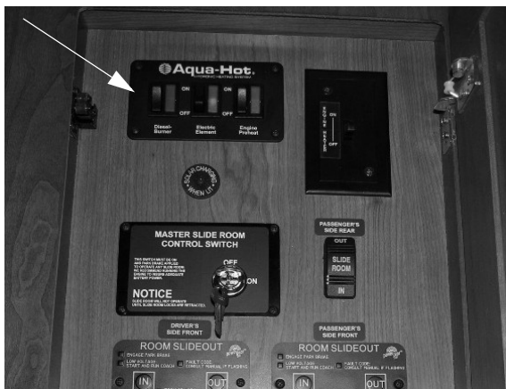
Hydronic Heating System Interior Control Switches (Located near monitor panel) -Typical View
