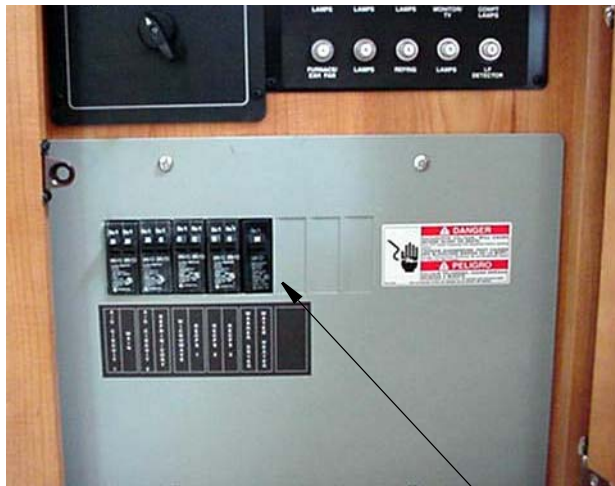
120-Volt House Circuit Breakers
