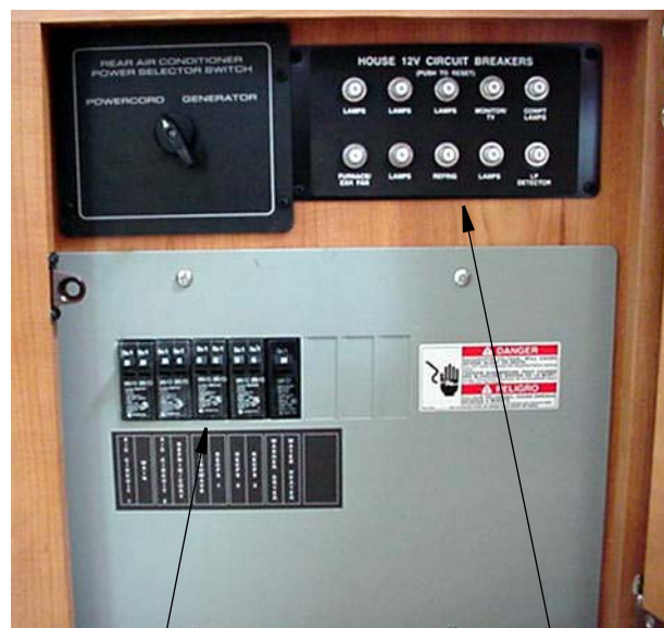
120-Volt House Circuit Breakers 12-Volt House Circuit Breakers Power Center (32' models)
