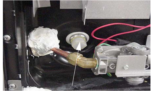
Water Heater Drain Plug (Remove with socket)
