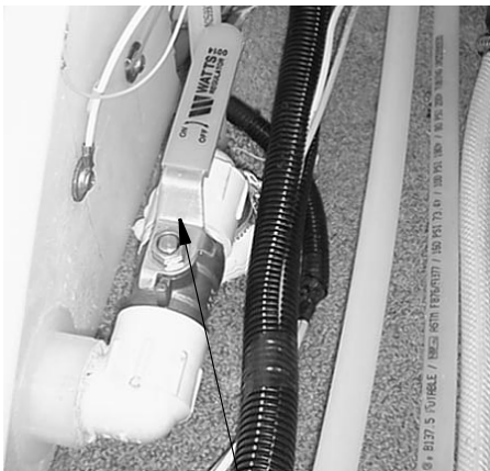
Water Tank Drain Valve (Typical)
