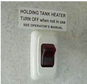
Holding Tank Heater Switch (Located near the monitor panel) -Typical View
