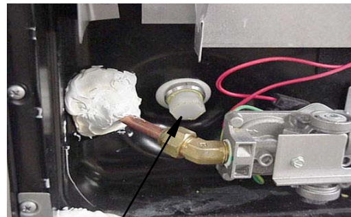
Water Heater Drain Plug (Remove with socket)
