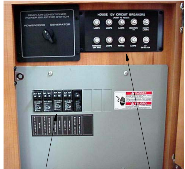
120-Volt House Circuit Breakers
