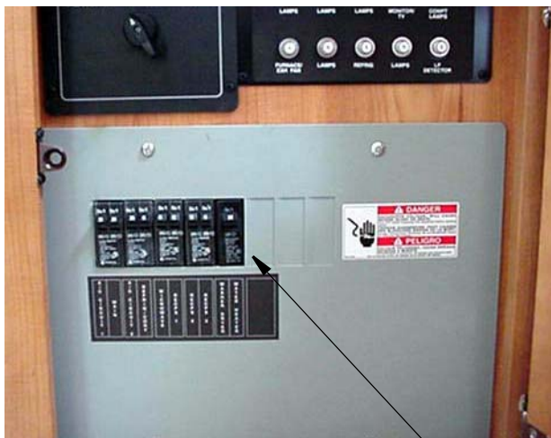
120-Volt House Circuit Breakers -Typical View
