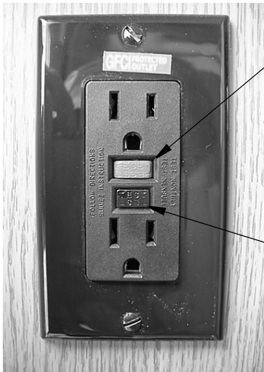
GFCI Outlet (Ground Fault Protector)
