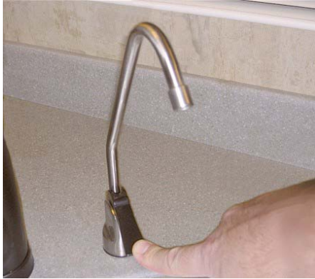
Filtered Water Faucet
