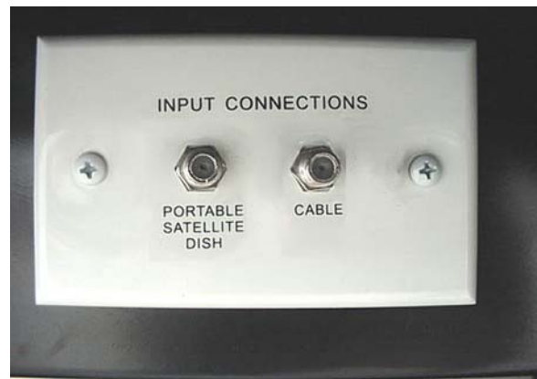
Exterior Connection for Satellite Dish and Cable TV (In Utility Compartment)
