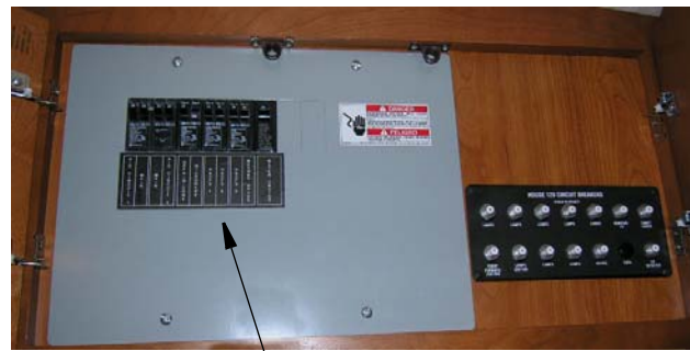
House 120-Volt AC Circuit Breaker Panel
