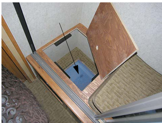
AC/Furnace Filter (Located under wardrobe floor panel) - Filter Size: 16" x 20"
