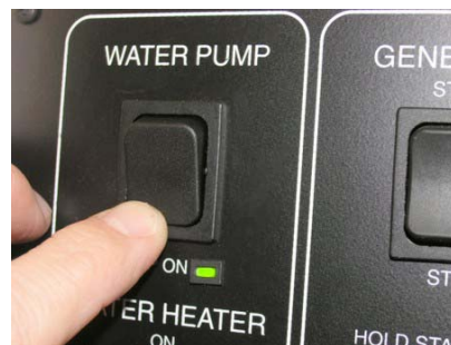
Water Pump Switch
