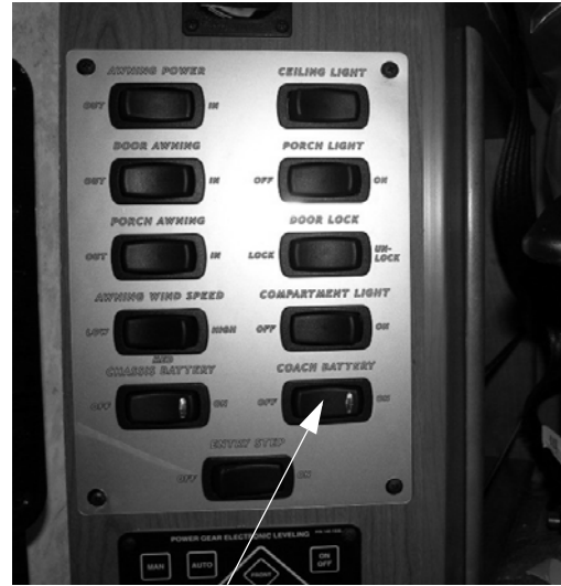
House/Coach Batt Disconnect Switch (Located near entrance door) -Typical View
