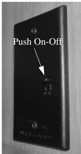
TV Signal Amplifier Power Switch -Typical View
