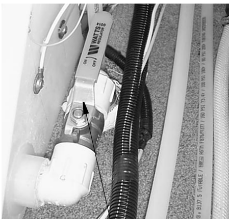
Water Tank Drain Valve (Typical)
