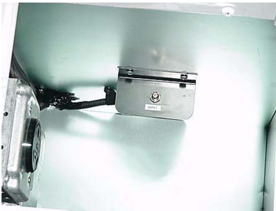
Cable TV Hook-Up in Utility Compartment
