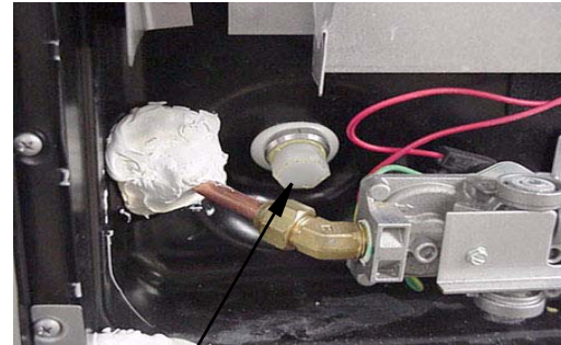
Water Heater Drain Plug Remove with socket.
