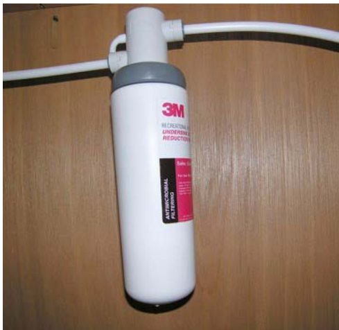
Water Filter Assembly (below Galley Sink)
