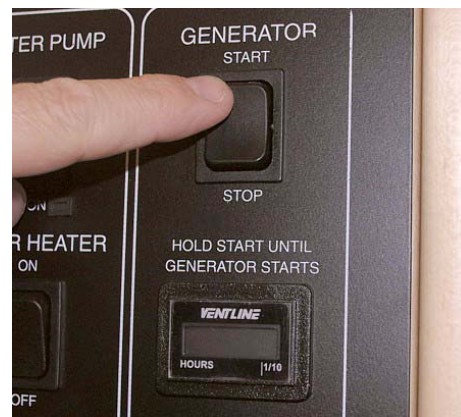
Generator Switch and Hourmeter on monitor panel
