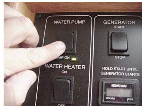
Water Pump Switch on OnePlace Panel
