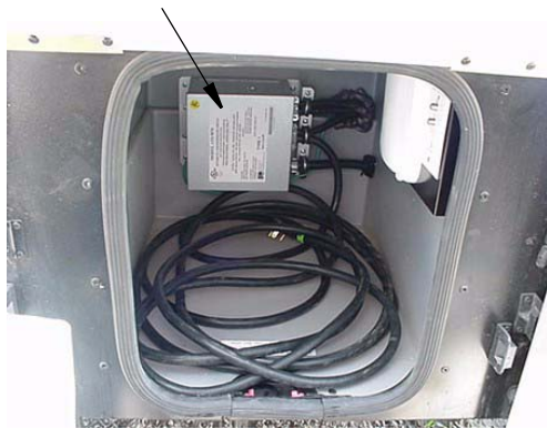
Power Transfer Switch
