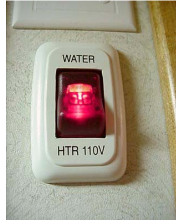
Electric Water Heater Switch (typically located near systems monitor panel)
