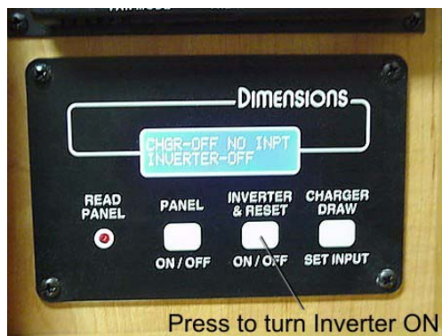
Inverter/Charger Control Panel
