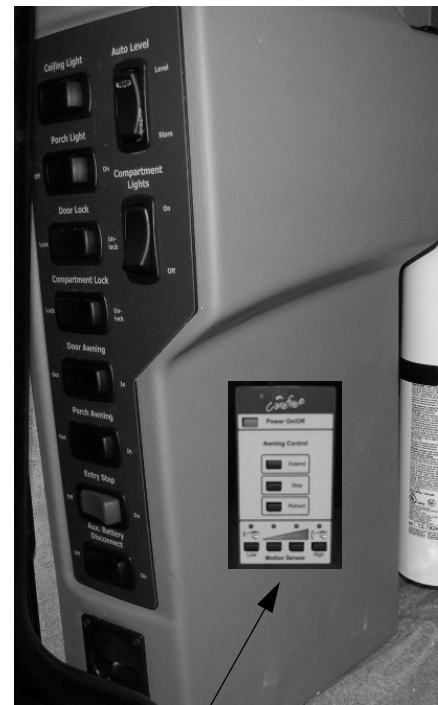
Awning Control Switch (Located just inside the entrance door)
