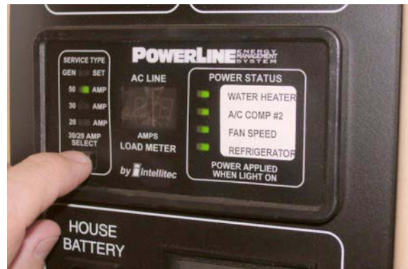
PowerLine EMS Display on Monitor Panel - Typical
