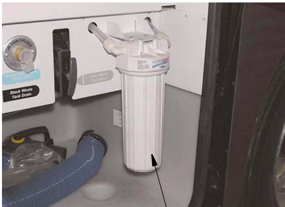
Full-Coach Water Filter System in Water Service Center (typical)
