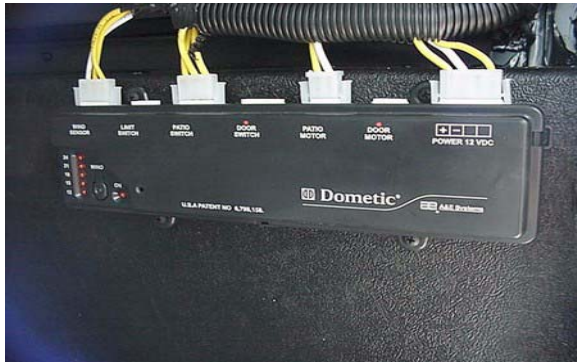
Awning Control Box (located in exterior compartment)
