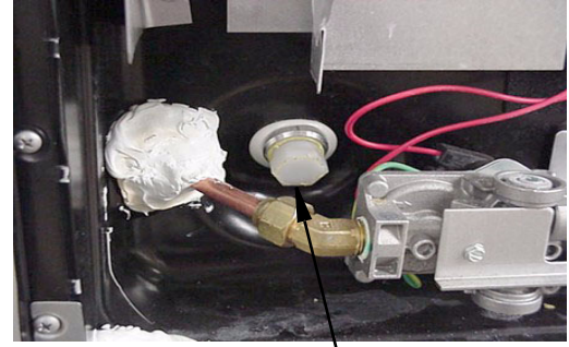
Water Heater Drain Plug Remove with socket.
