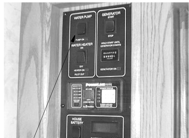
Water Pump Switch
