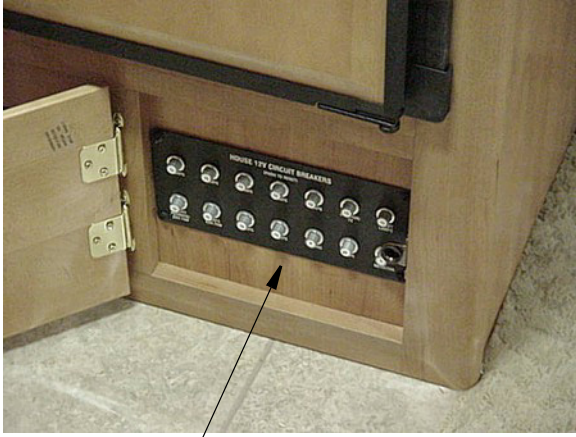
House 12-Volt Circuit Breaker Panel - typical*
