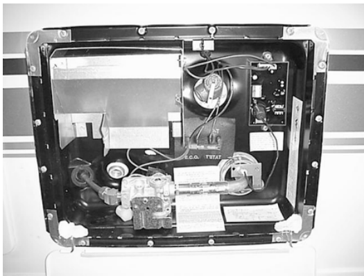
Water Heater Exterior Service Access
