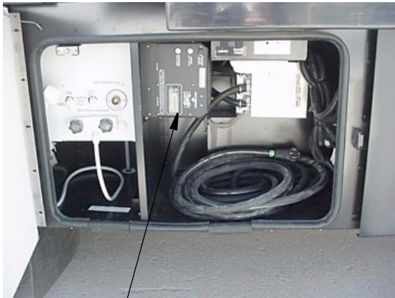
Inverter Charger Unit Location in utility compartment
