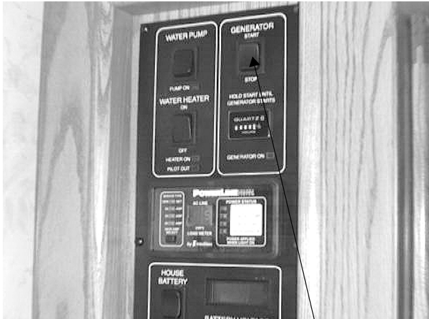
Generator Switch and Hourmeter
