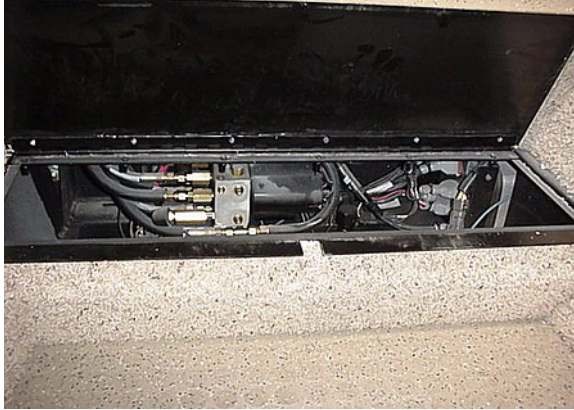
Hydraulic Pump beneath Entry Step
