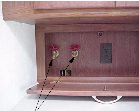
Water Supply Faucets -typical
