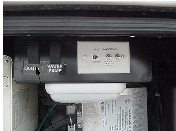
Utility Light Switch
