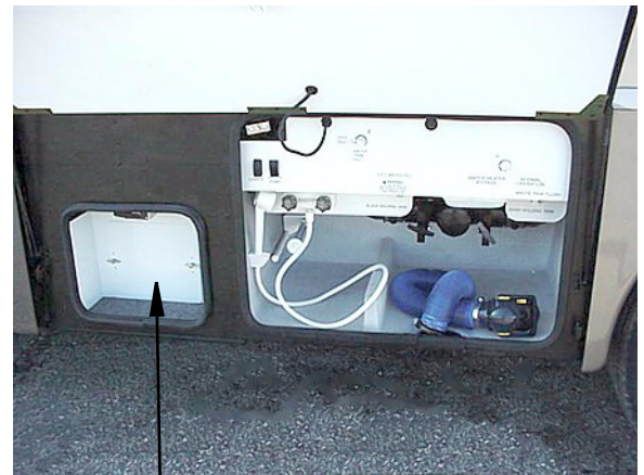
Water drain valves located behind access panel
