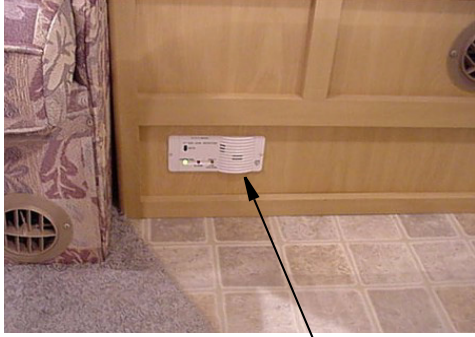
LP Gas Leak Detector
